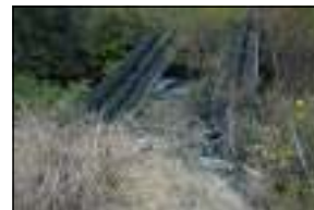
A burnt out bridge
